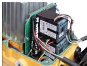
LOW VOLTAGE CONTROL
